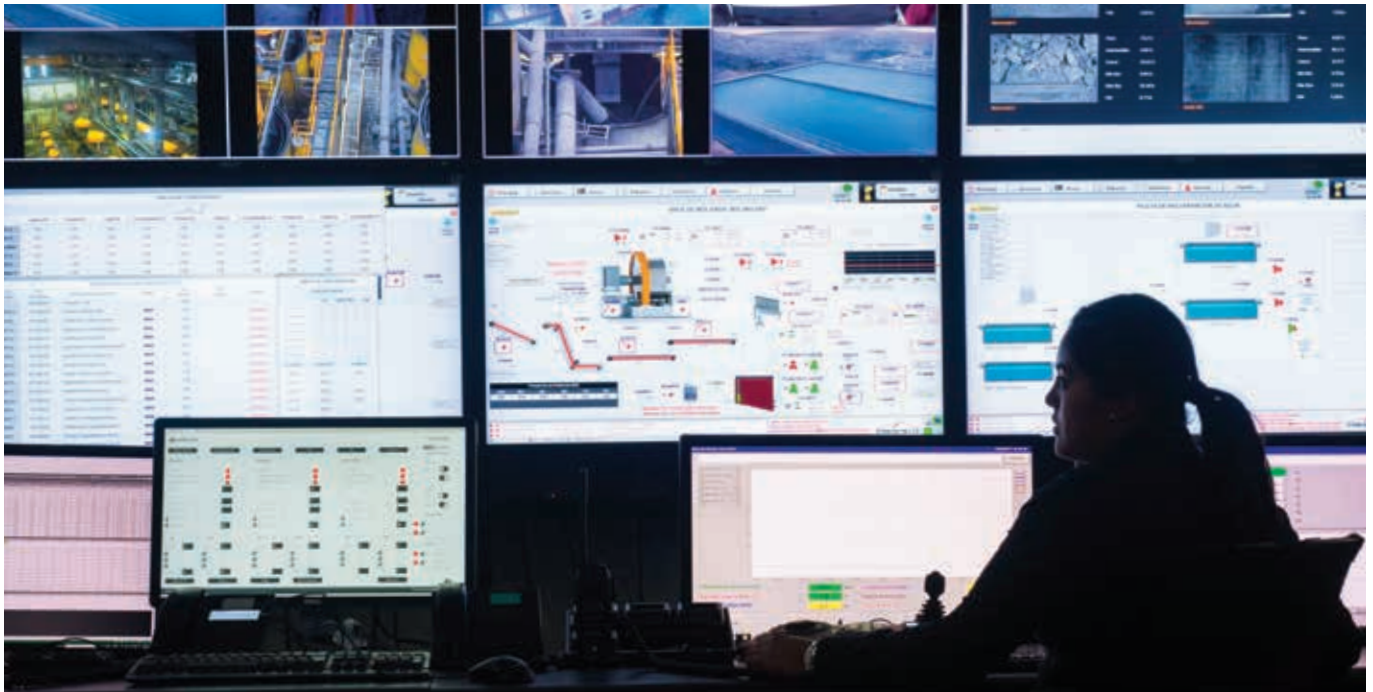
Saucito control room
