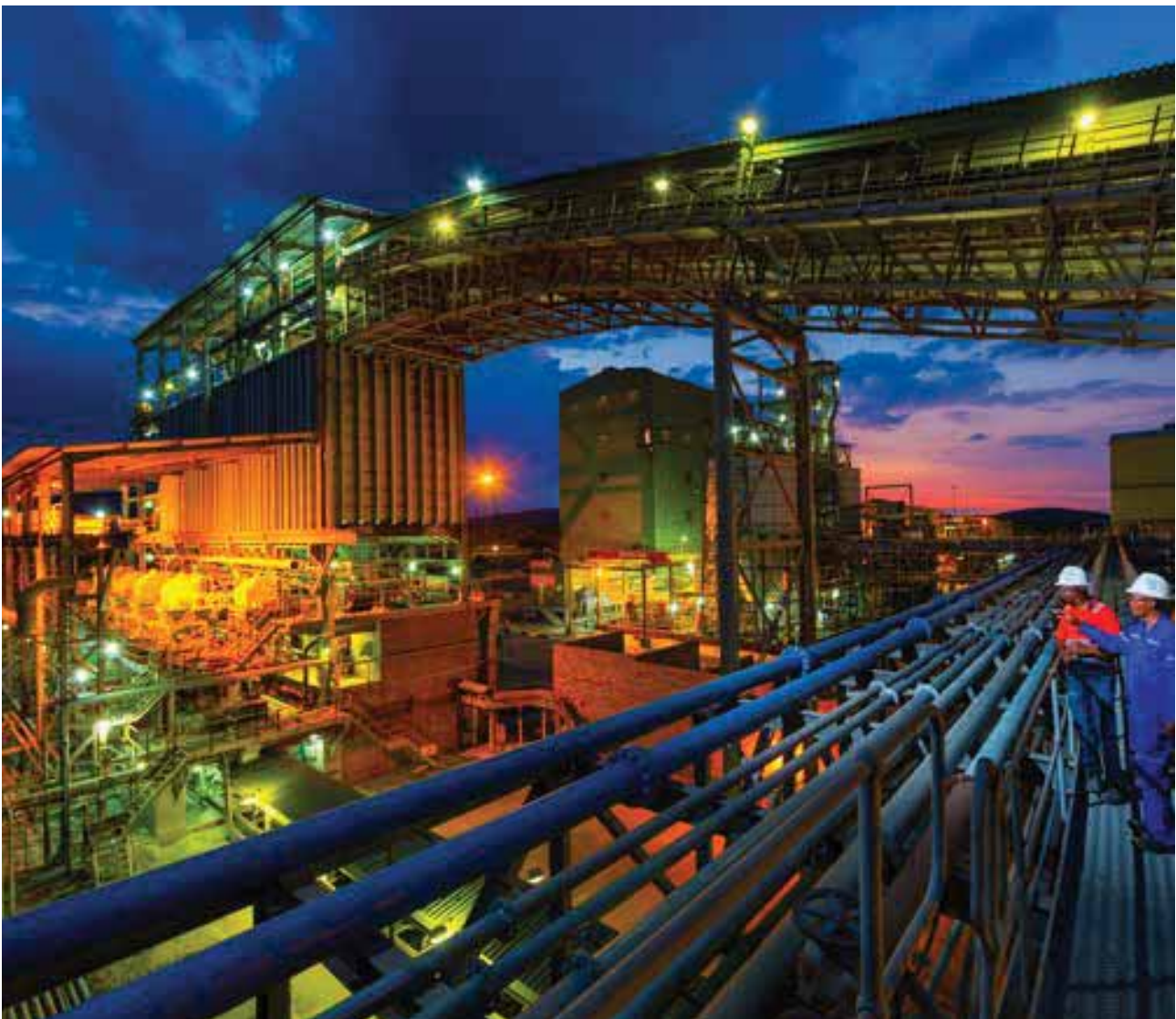
The BRPM concentrator which was upgraded to 250ktpm in 2016
