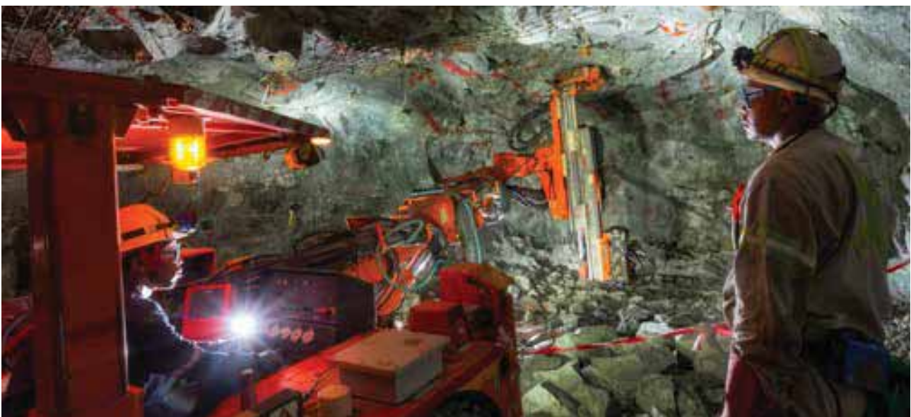
Miner overseeing bolting of a newly blasted breakaway of 600 level at Styldrift I
