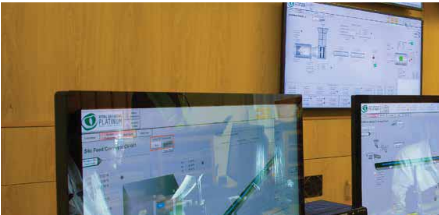
The control room at Styldrift I, mechanised mine.
