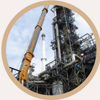
Figure1: Continuous Catalyst Regeneration Platform Unit - 1
